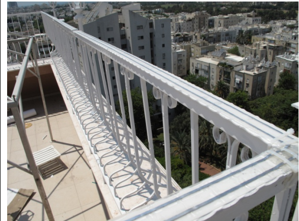
Figure 7. Bird Stop™ Electric Tape protecting a handrail. Photo by Bird Stop™ USA.
